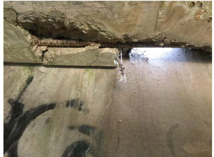
Damage to deck panel on right bank
