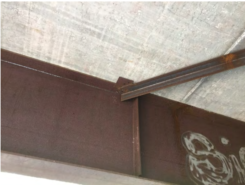
Bracing at right bank missing bolts but welded
