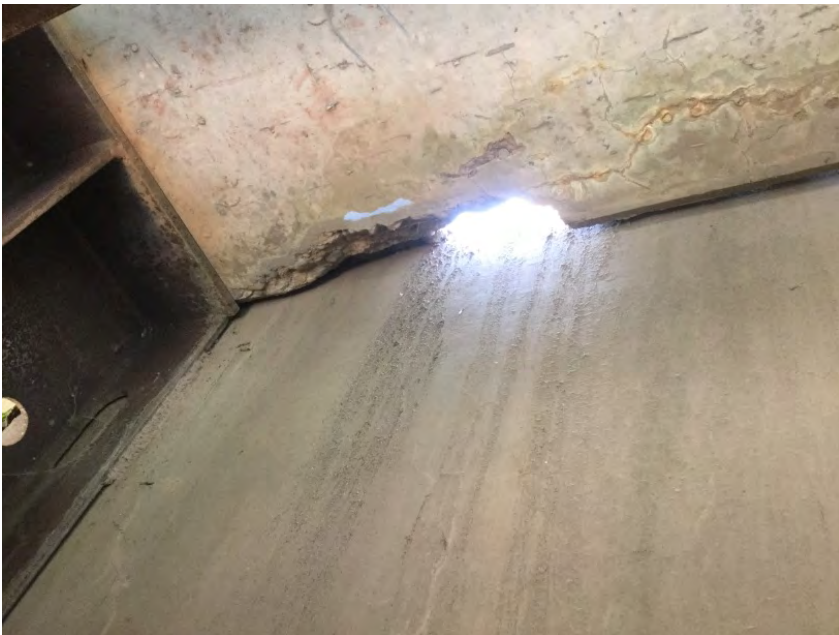
Damage to panel at left bank
