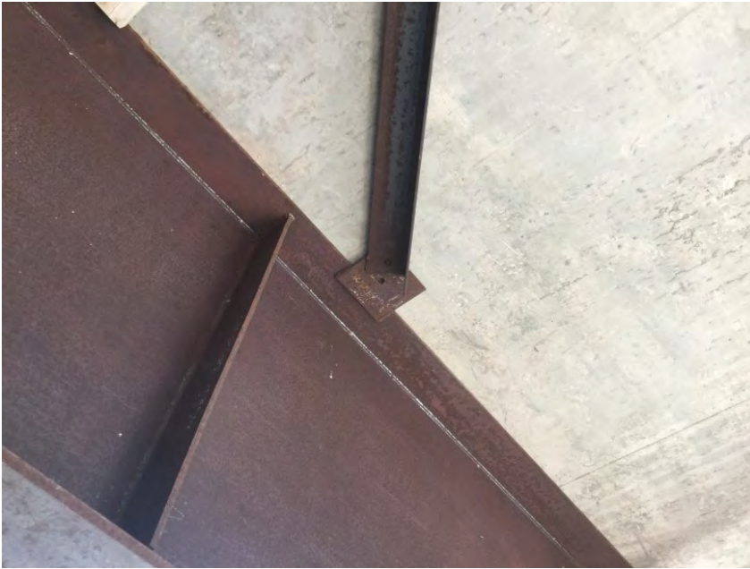
Bracing at left bank missing bolts but welded
